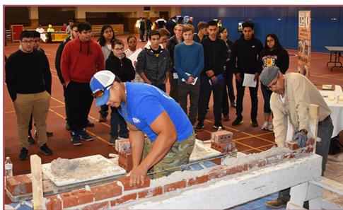
Bricklayers' 2nd-year apprentice Chris Winston (left) and Instructor Isidro Valdez demonstrate laying brick to students.
