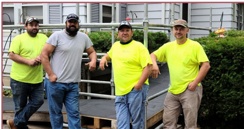
Laborers who worked on the ramp (from left) are Alex Tucker (68), Enrique Cardenas (4), Chris Lezon (6) and Mariusz Zawada (4). Photos courtesy of Laborers Local 4.
