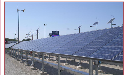
The solar panels at the IBEW-NECA IN-TECH Renewable Energy Training Field.
