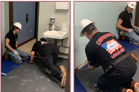
Carpenters from Local 1185 work on the floors and baseboards of one of the rooms at the Gateway to Learning Training Center in Chicago.
